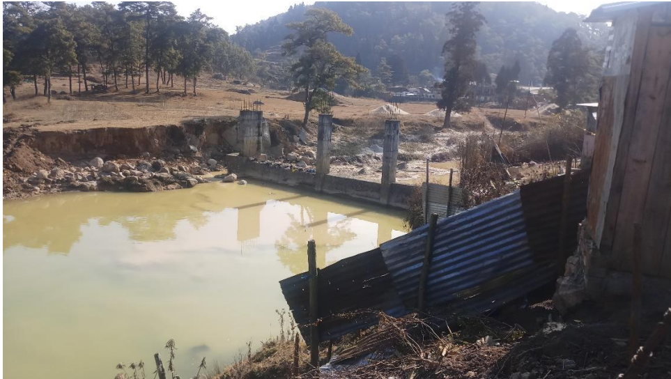
Figure 17 Flash floods washed away shoulders of silt trap (Umiew and Umtyngar rivers)
